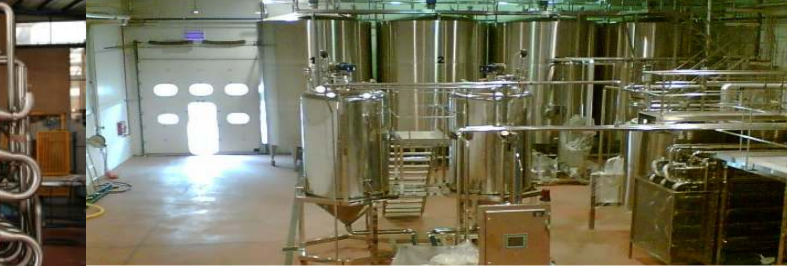
Storage and mixing tanks
