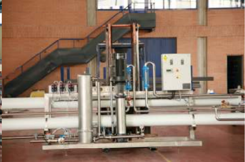
Reverse osmosis unit
