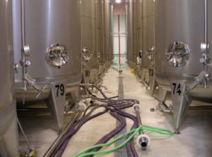
Aseptic storage tank
